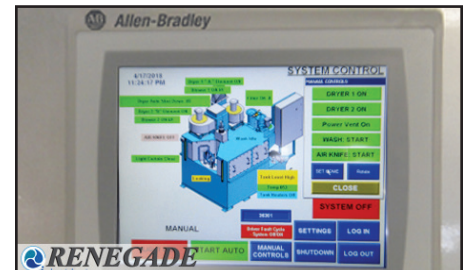
Allen-Bradley Monitor with Large, Touch Screen PLC/HMI Controls.
